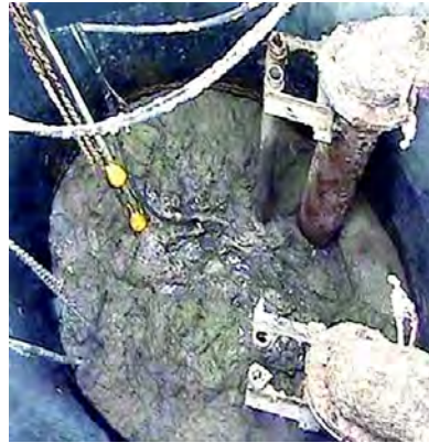
Before Treatment With the Little John Digester
