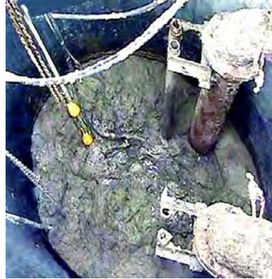
Before Treatment With the Little John Digester
